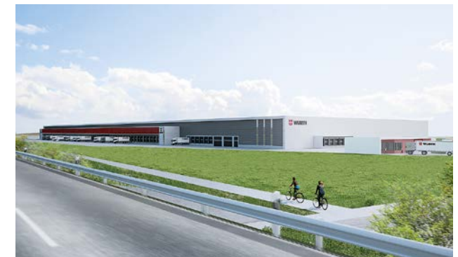
Under construction: new freight hub of Adolf Würth GmbH & Co. KG directly next to the A6
